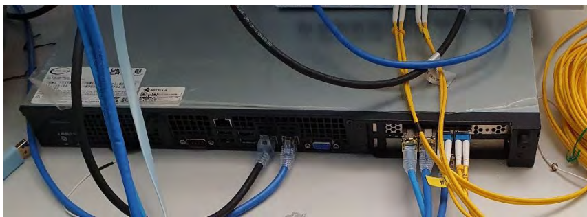
Figure 29: CU/DU Board (NXP Layerscape® Access processors) And 5GC Server compact implementation. Backhaul deployed over 10Gbit Ethernet.
